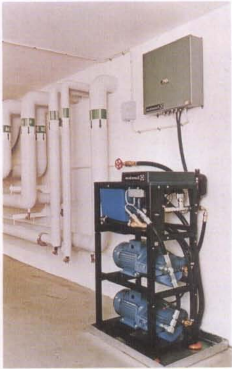
Central unit with high pressure pumps and automatic controls.
