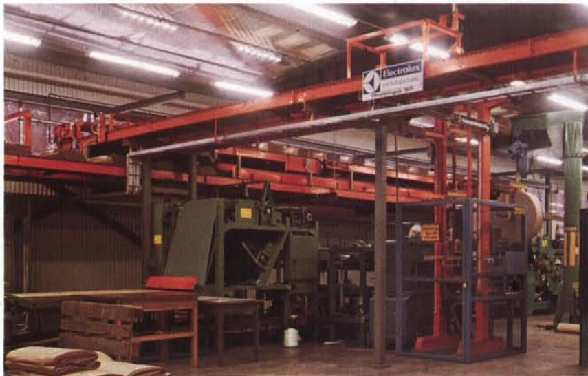
B. A vertical hoist connected with accumulating conveyors. The paper bags are piled automatically while waiting to be loaded on stools (see also sketch outline on page 18).
