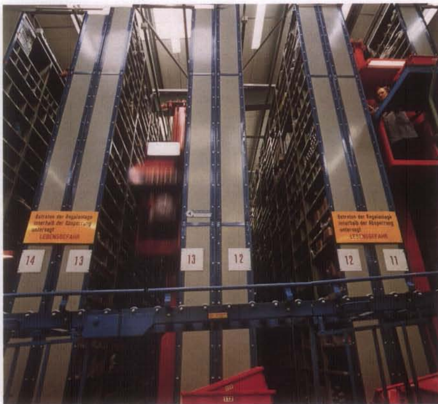
A materials handling installation delivered to the central spare parts store of Volvo Deutschland Vertriebsgesellschaft at Dietzenbach in Germany. The racks, 150 feet (45 m) long and 23 feet (7 m) high, hold 30,000 items. The installation also includes four manually operated picker cranes.
