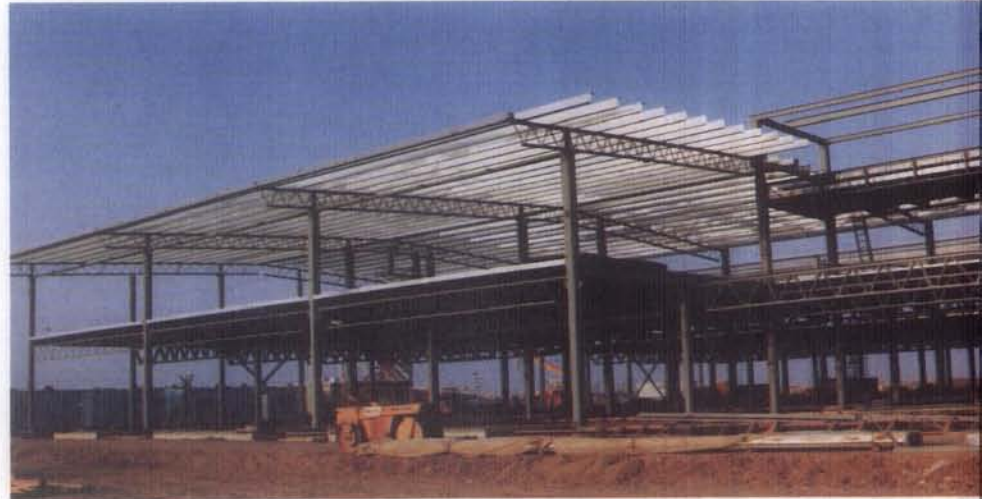
Gränges Hedlund supplied and erected the steel framework for the administration block in Jeddah's new airport. Other Gränges companies contributed building materials, aluminium sheeting and tubing.
