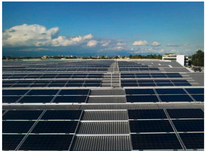
Solar panel roof of the facility in Vallenoncello.
