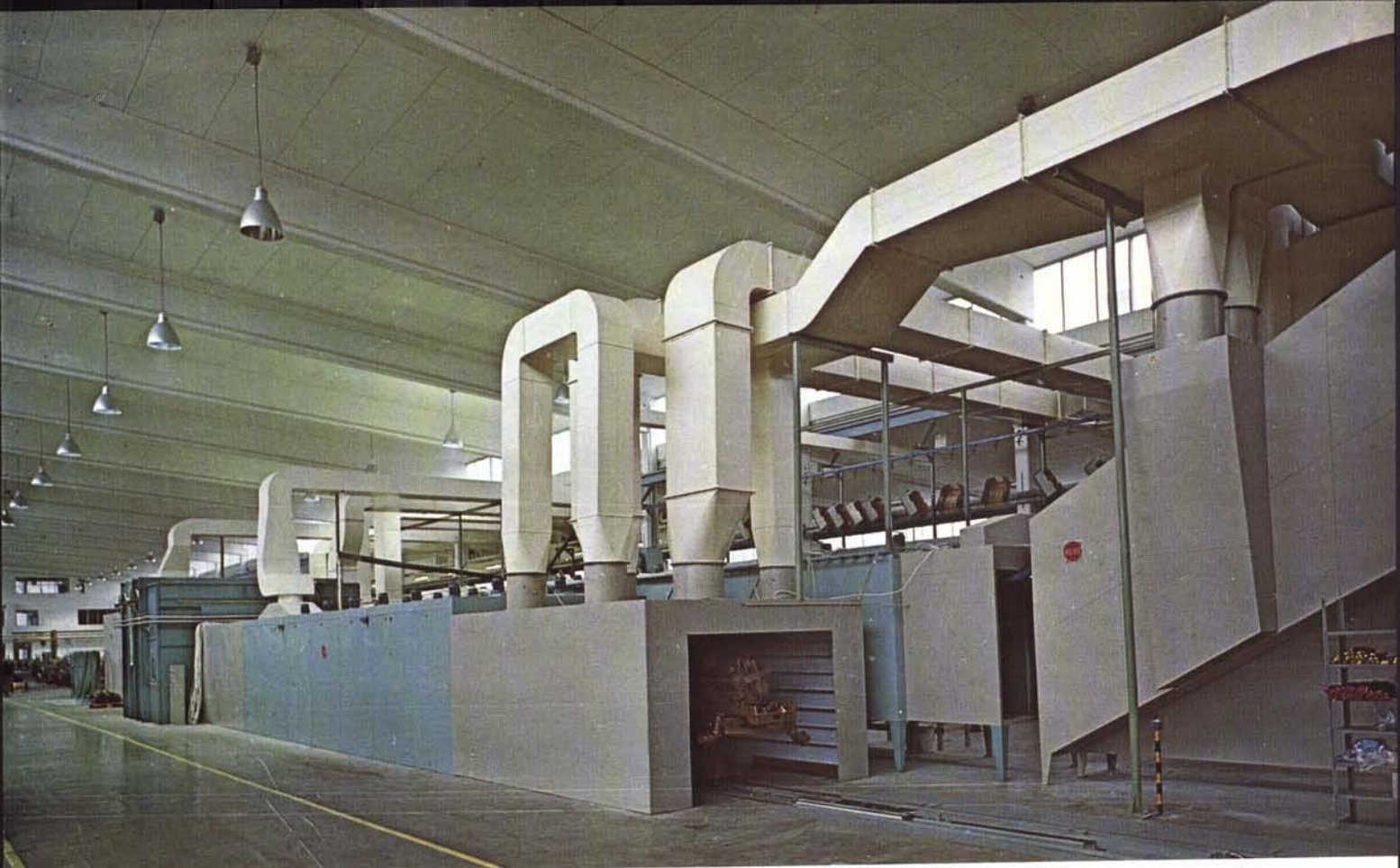
A drying plant, manufactured by the Electrolux Alingsås factory and installed at the Valmet OY tractor factory at Jyväskylä, Finland.
