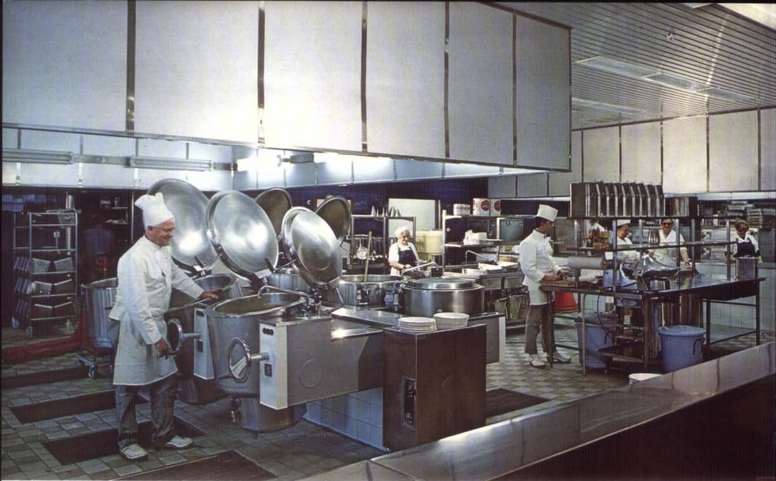
Electrolux are specialists in catering equipment. This picture shows an installation at Telefon AB L. M. Ericsson, Stockholm.
